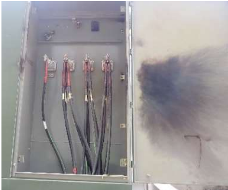
2.23: Damage upon transformer due to arc flash accident
