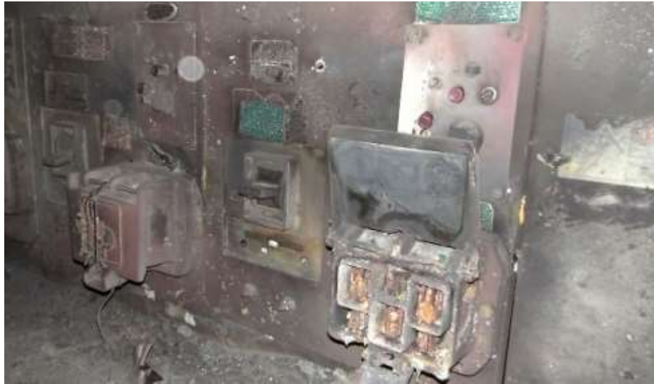
2.22: Aftermath of burnout breaker after arc flash accident
