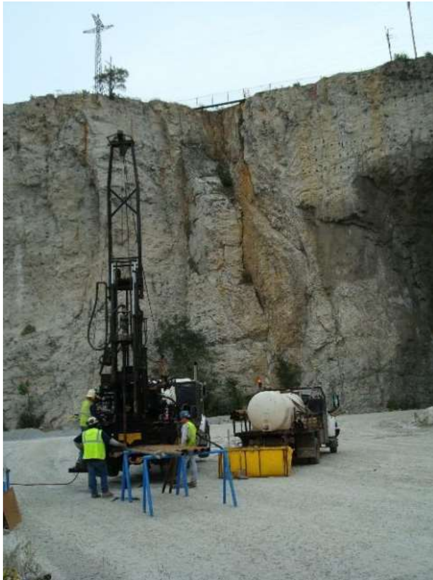
4.8: Using drills responsibly in both above-ground and underground mining is crucial for efficiency and production and essential for safety and hazard prevention
