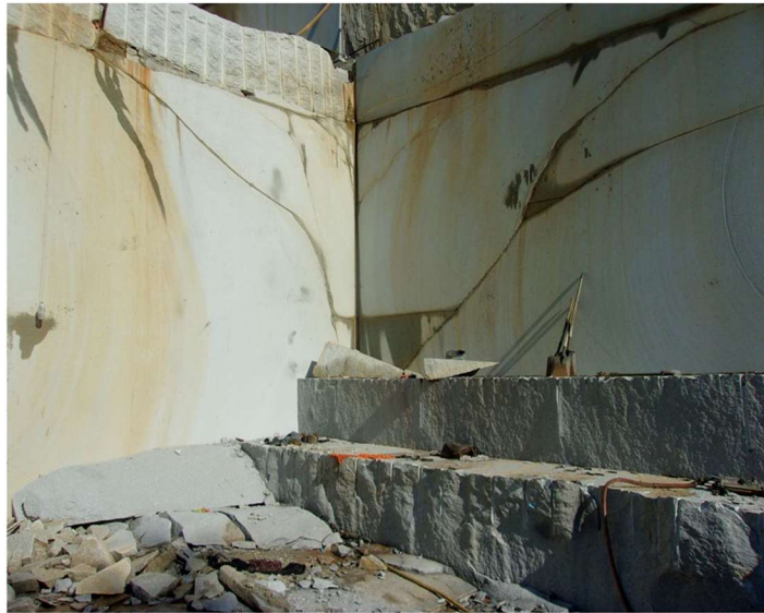
4.7: An accident from loose quarry material occurred because the mine operator did not correct hazardous ground conditions
